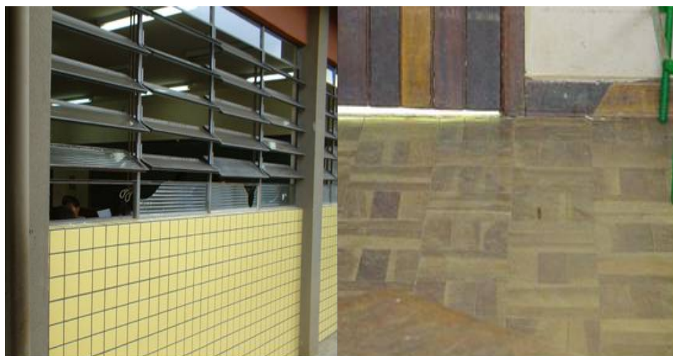
Fig. 18. Classroom com broken window panes and spaces between the door and the floor
