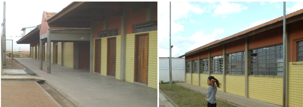
Fig. 17. Façade of a classroom – left: Door and Walls; right: Wall and Windows
