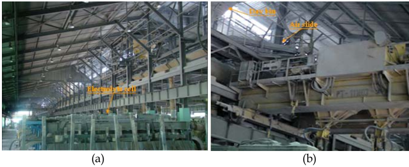
Fig. 2. a) Aluminum smelter pot room, b) Overhead crane being fed of alumina from a day bin by a standard air slide.
