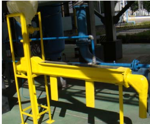
Fig. 20. Air-fluidized conveyor of 1.5 m long with three outlets.
