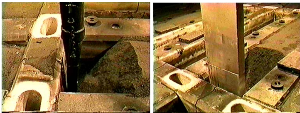
Fig. 14. Albras bake furnace coke suction system before and after modifications – source: Albras Alumínio Brasileiro SA.
