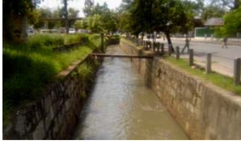
Fig.12. Canalised Joana River stretch, in Rio de Janeiro City, Brazil
