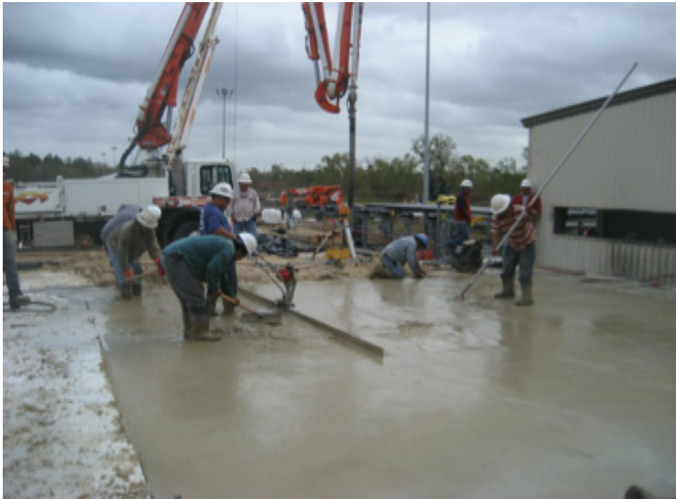
Fig. 4. Construction of base for a heat treating facility in Houston, Texas. Cycling of temperatures caused severe breakdown of conventional concrete, (James K. Hicks, et. al., 2009).
