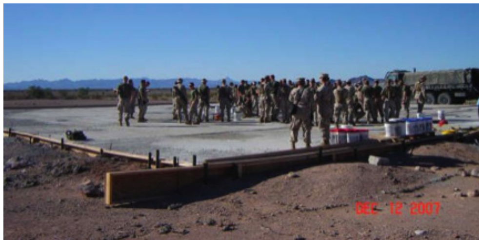
Fig. 5. Marine Corps Engineers training for fast track construction and repair prior to deployment. Marine Corps Base Concrete Installation, (James K. Hicks, et. al., 2009).
