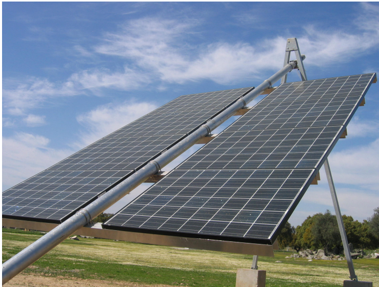
Fig. 4. Solar Park - motorized PV panels
