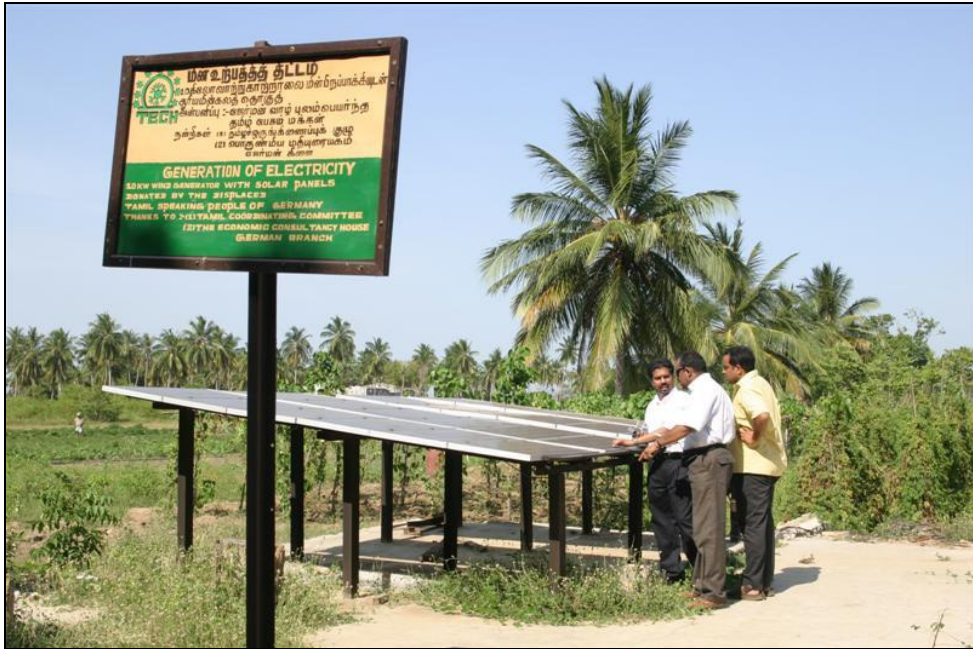
Fig. 2. Solar panel installed in NE-SL
