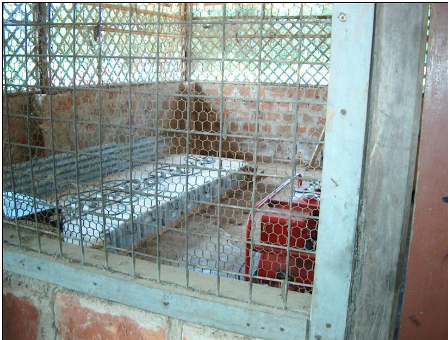
Fig. 4. Battery Storage System
