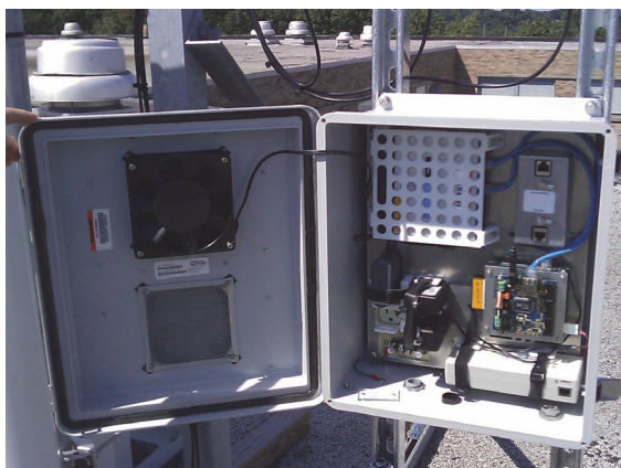
Fig. 10. Electronics equipment supporting prototype subscriber stations during testing.
